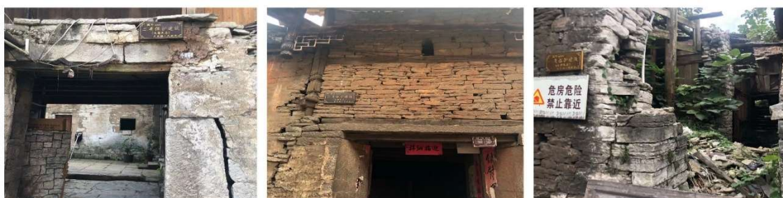
Figure 2. The status quo of some traditional buildings in Tunpu village
